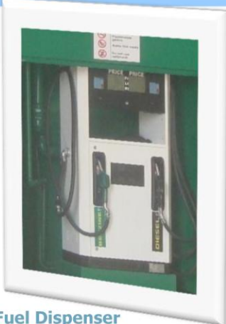
Fuel Dispenser dispensing niche with gas pump
